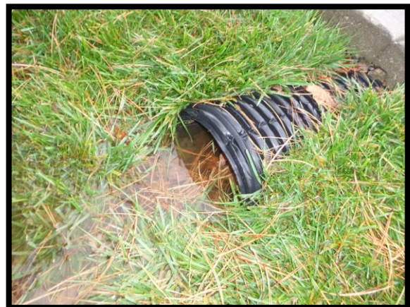
Evidence of ponding water within the underdrain pipe draining the swale.
