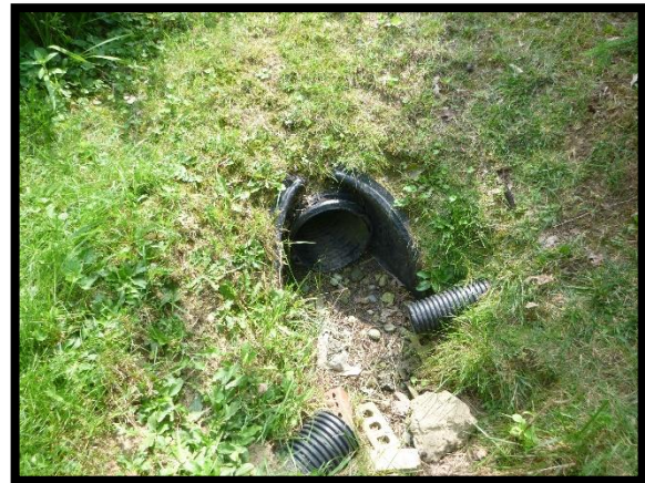
View of 12-inch CPP outlet pipe that drains east to the 36-inch Robinwood trunk line.
